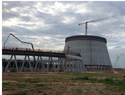
Fig. 9 Power plant cooling tower
